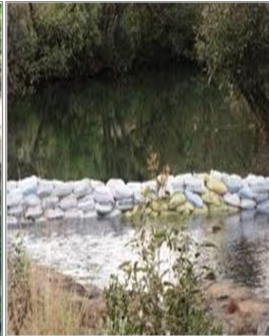
Fig 4: Loose boulder wall
