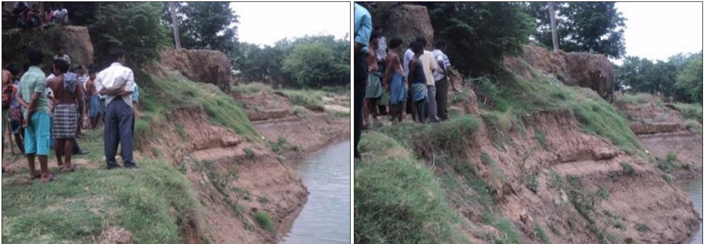
Fig 5: Land Sliding of Shilabati River at Haldighat under Dewanchak – II Gp
