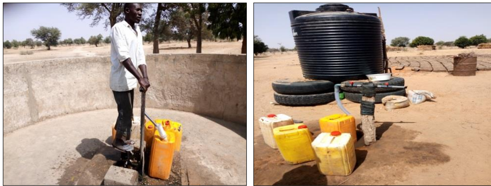
Foot pump borehole
